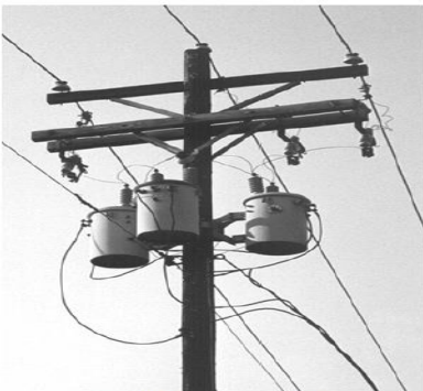
Figure 5-18 Three-phase transformer bank.
